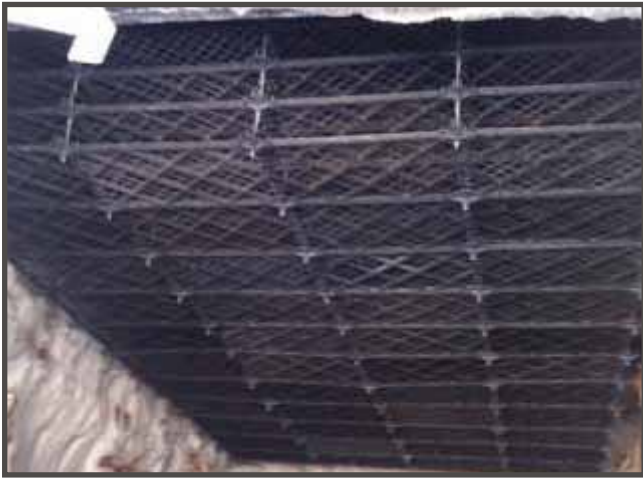
Refurbishment of the Old Cooling Tower with a new type of packing
