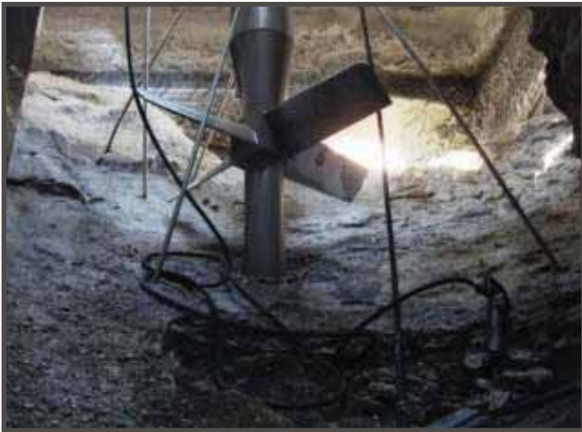
Build up of hard material (similar to concrete) inside Reactor
