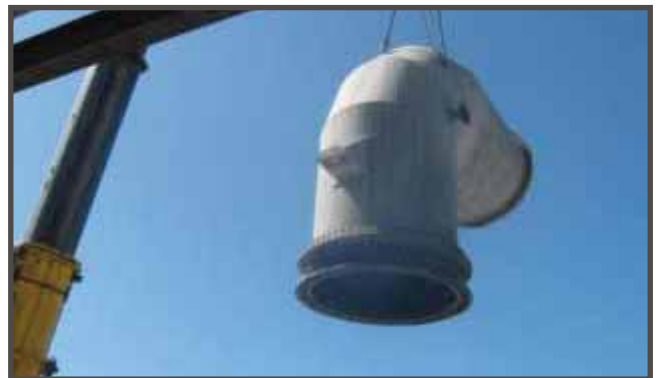
Acid duct being removed in New Phos. Conc. for Heat Exchanger Seal repair
