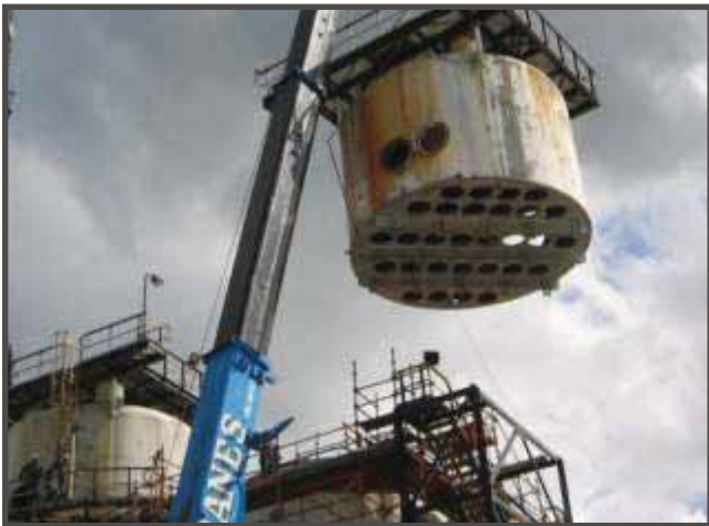
New Candle Plate welded to head section of Inter-pass Tower being re-assembled
