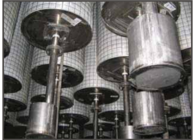
Candle Filter replacement in the Final Absorption Tower
