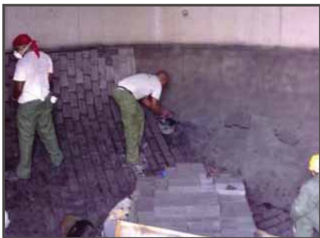
Carbon brick lining in Evaporator
